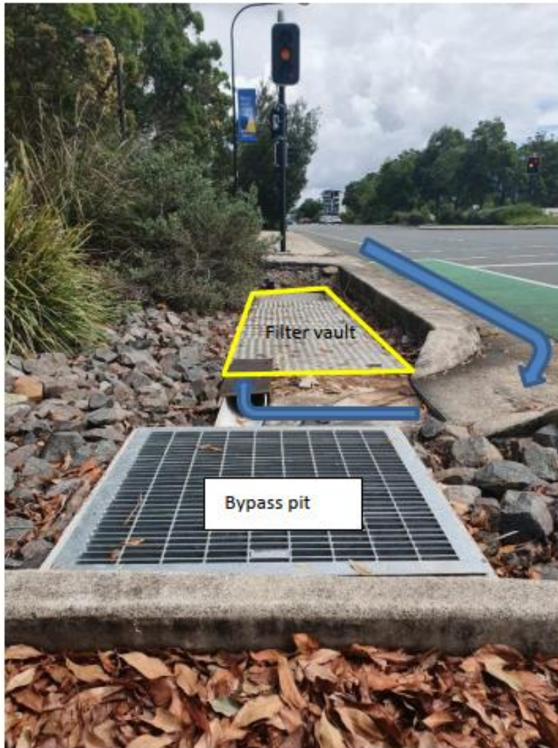
Figure 4: Sippy Downs Half Height Monitoring Equipment Arrangement
