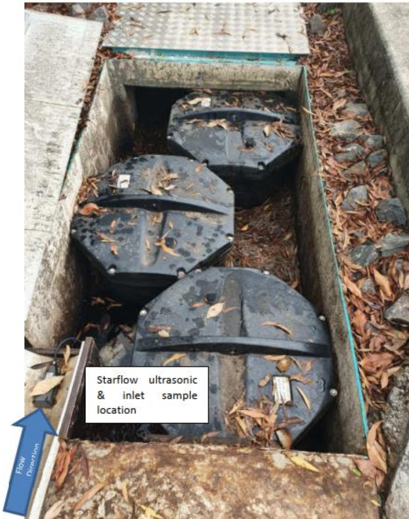
Figure 3: Sippy Downs Drive Filter Vault
